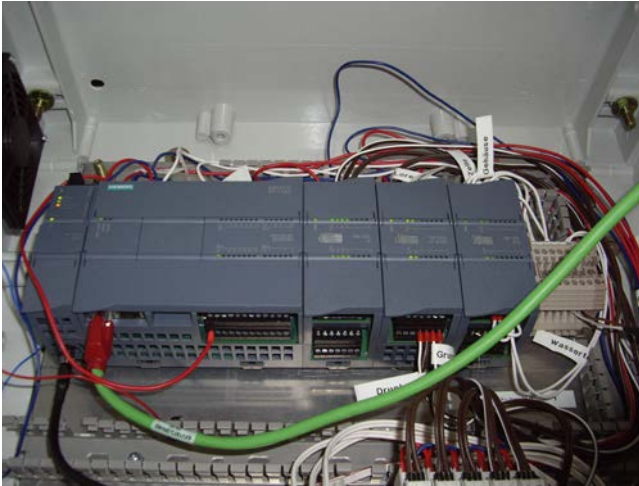
TeleControl Basic telecontrol technology from Siemens is used to monitor and control the remote systems in Nicaragua.
